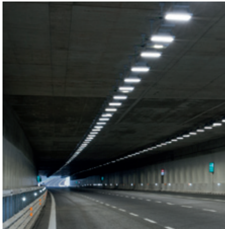
Tunnel interior lighting
